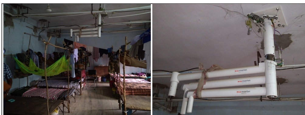
Photograph taken on 04 October 2019 showing proposed Operation Theatre of the Dental Institute and incomplete installation of OT Light.
